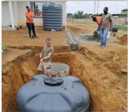
"Installation of rainwater harvesting tank at Chitungwiza Swiss House. This technology may become a model for similar future projects."
