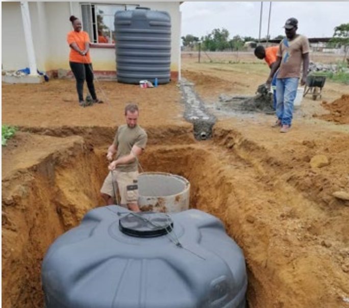
“ Installation of rainwater harvesting tank at Chitungwiza Swiss House. This technology may become a model for similar future projects.”
